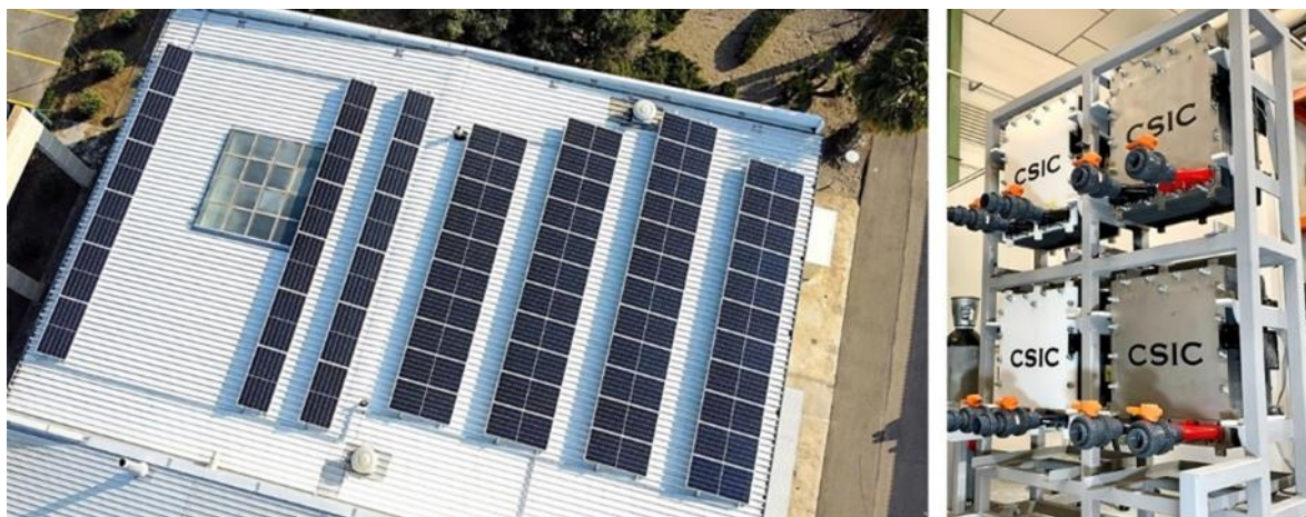
Photovoltaic panels from the solar field mounted on the roof deck of the main LIFTEC building (left). 10 kW VRFB designed and fabricated in the framework of FLOWBAT works (right)
